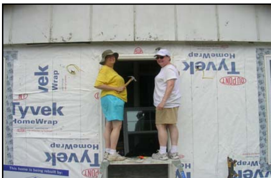
Kate Chambers (Academy of the Holy Angels) & Sr. Maria Iannuccillo, SSND working on siding.
